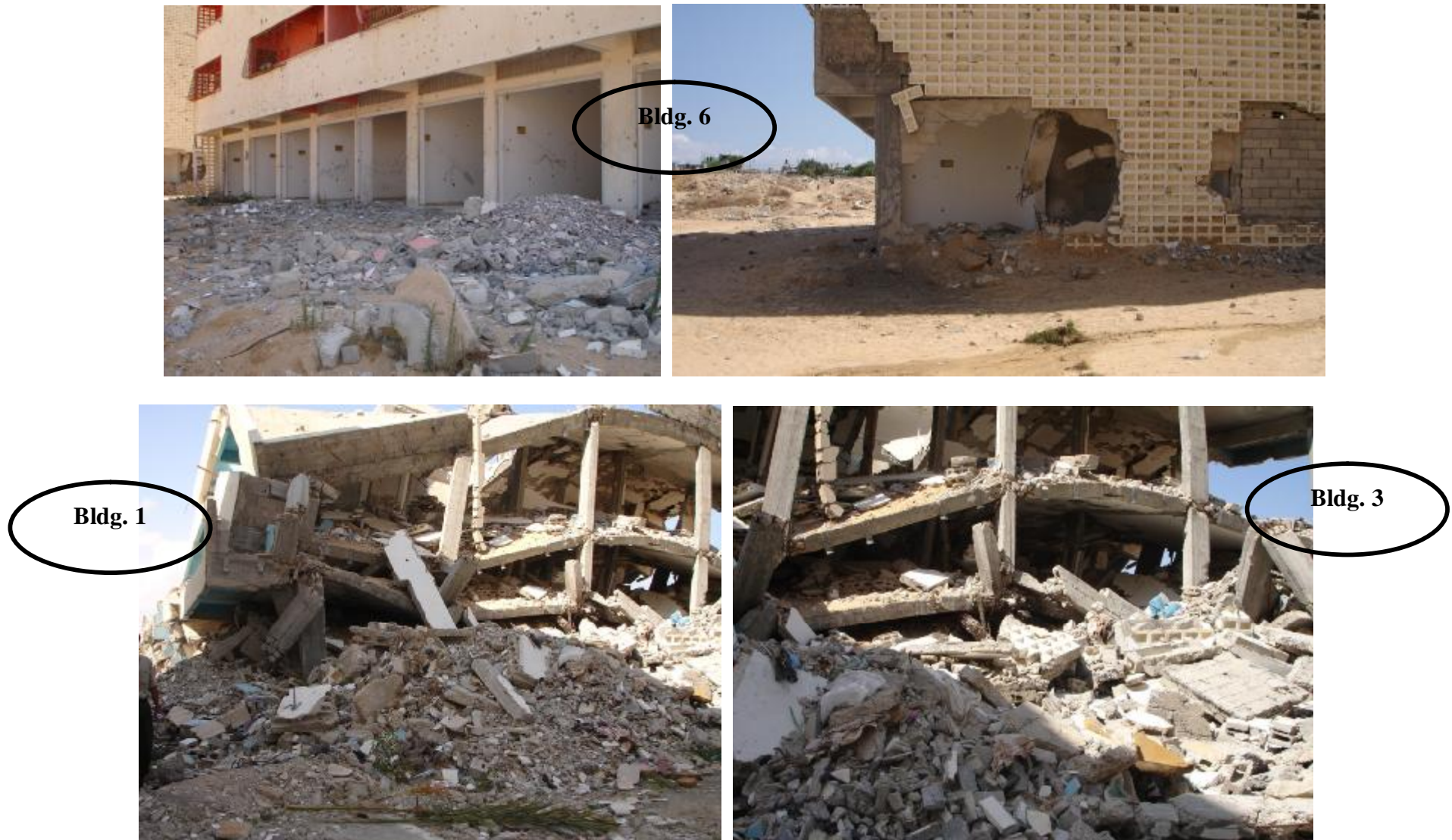
Figure S-7: Damages to the AHP during EL-Aqsa Intifada
